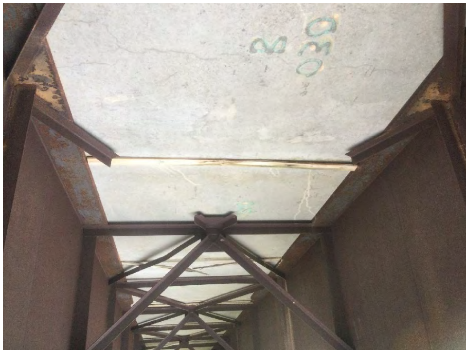
Photo 26 Missing plan bracing near mid-span
