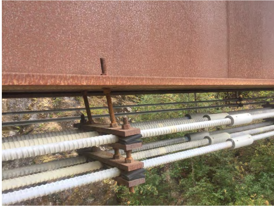
Photo 27 Downstream hangers angled
