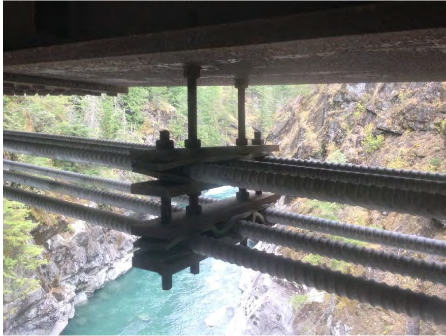
Photo 21 Typical hangar and rod condition
