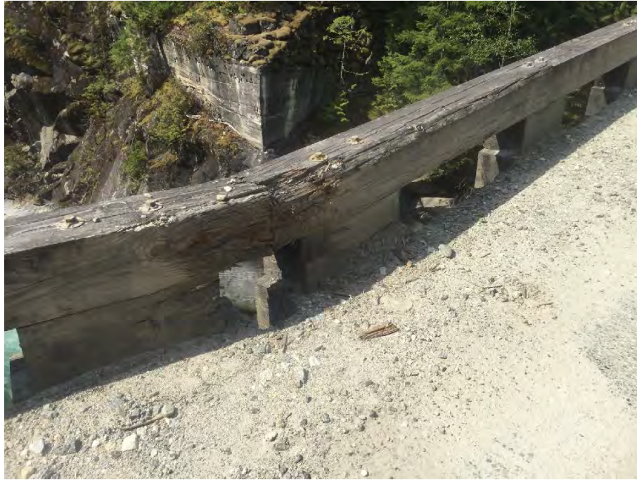
Photo 25 Downstream railing damage at flare corner
