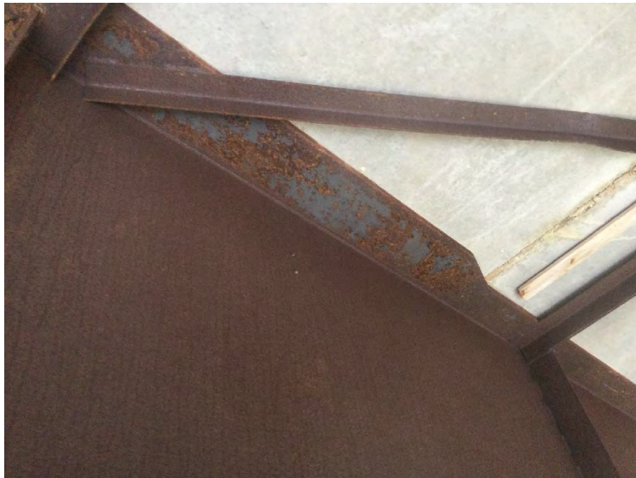
Photo 28 Typical top flange corrosion
