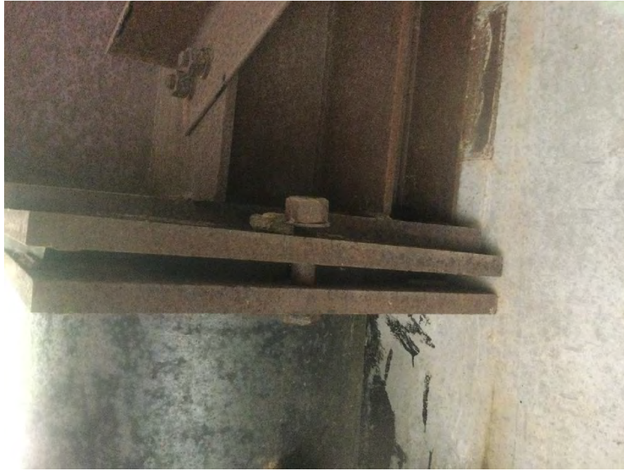
Photo 29 Failed anchor bolt
